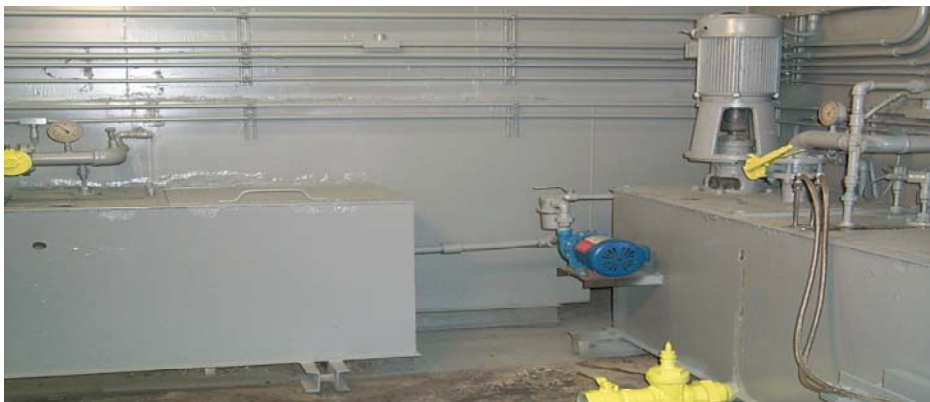
Figure 6. Rinse Counterflow System
